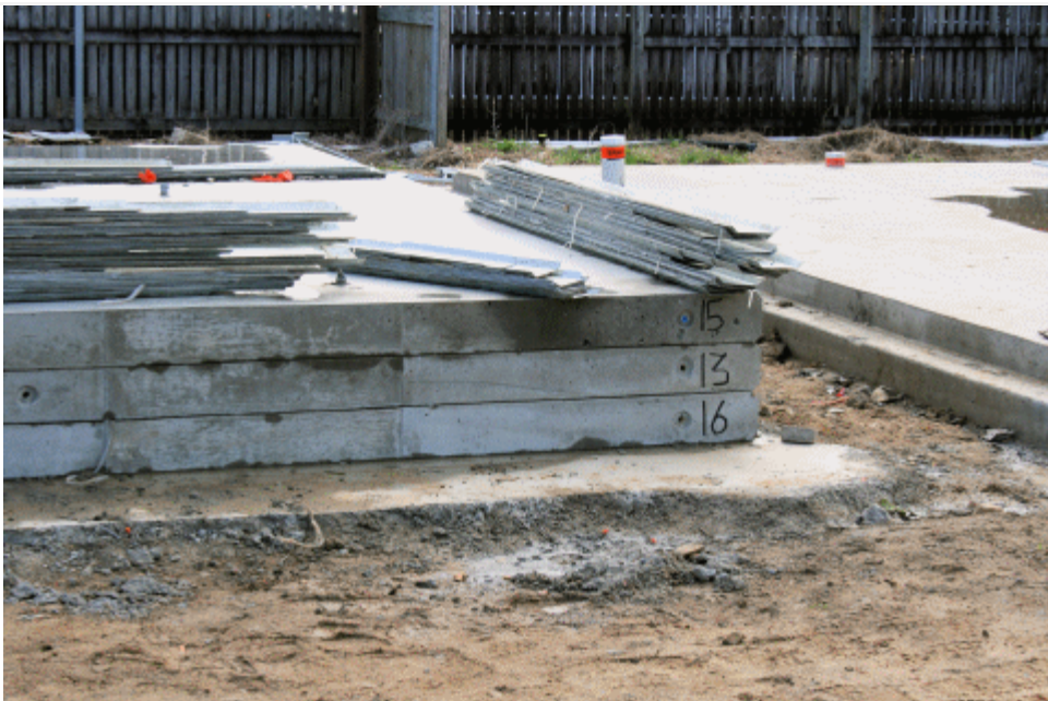
More stacked panels. Note the numbering – each panel has an ID number and a lift sequence so that they are lifted in the correct order. These were poured on a temporary slab of concrete next to the building which will be removed later.
