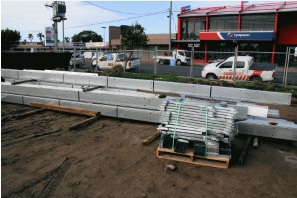
The first of the structural steel has been delivered. These are roof purlins.
