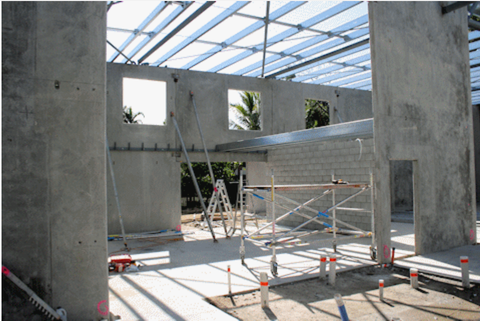
Looking past the toilets to the crèche room. The cross beams are the support for the mezzanine floor.
