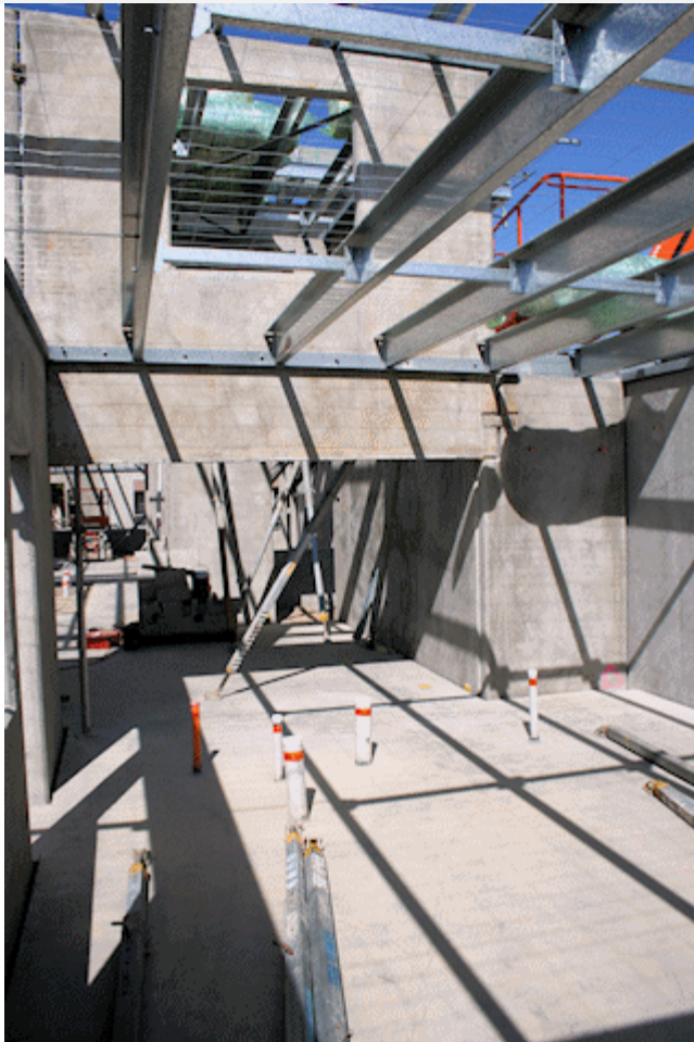
Standing in the corner of the kitchen looking towards the crèche room. Note that the space you see will be filled with cupboards facing the crèche room and a food storage room for the kitchen.
