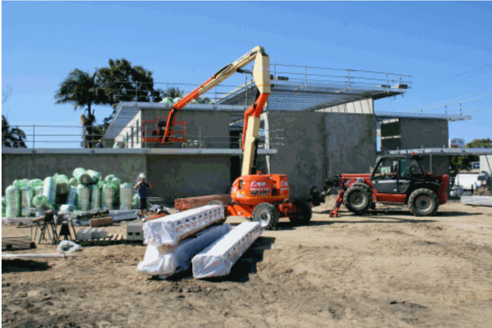
Front of the building, with insulation and roofing materials being lifted into position. Framework above the roof are temporary safety scaffolding.
